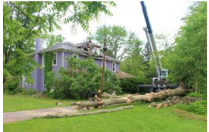
Oberlin House after a 70' tree fell through the roof
